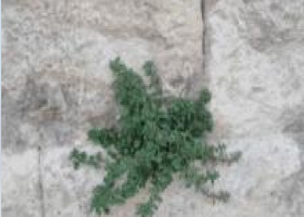
Eroded of stone surfaces due to botanical and microbiological effects, depending on accumulated pollutants
