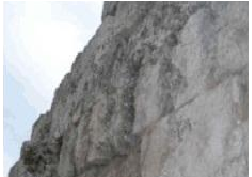
Discolouring of some zones on the stone surfaces due to soot, dirt, and impurities of polluted oxides
